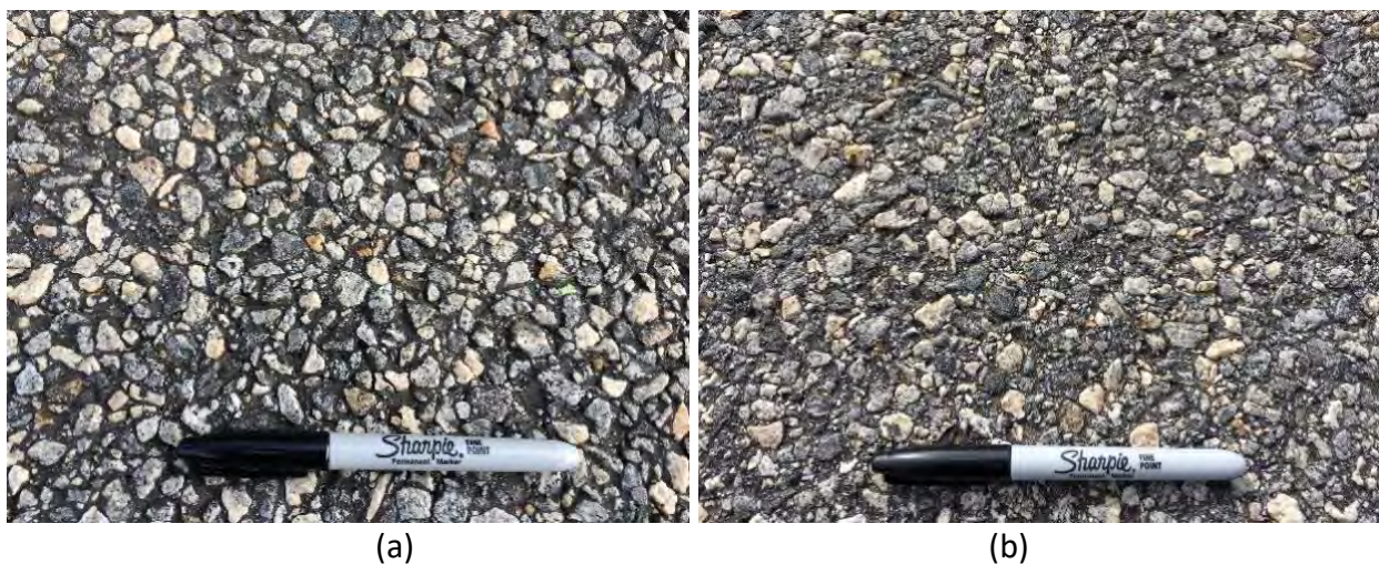
Figure 39. NCAT Test Track Pavement Sections; (a) SMA, (b) Polymer-Modified Superpave Dense-Graded Mixture (Photos Taken in June 2017)
